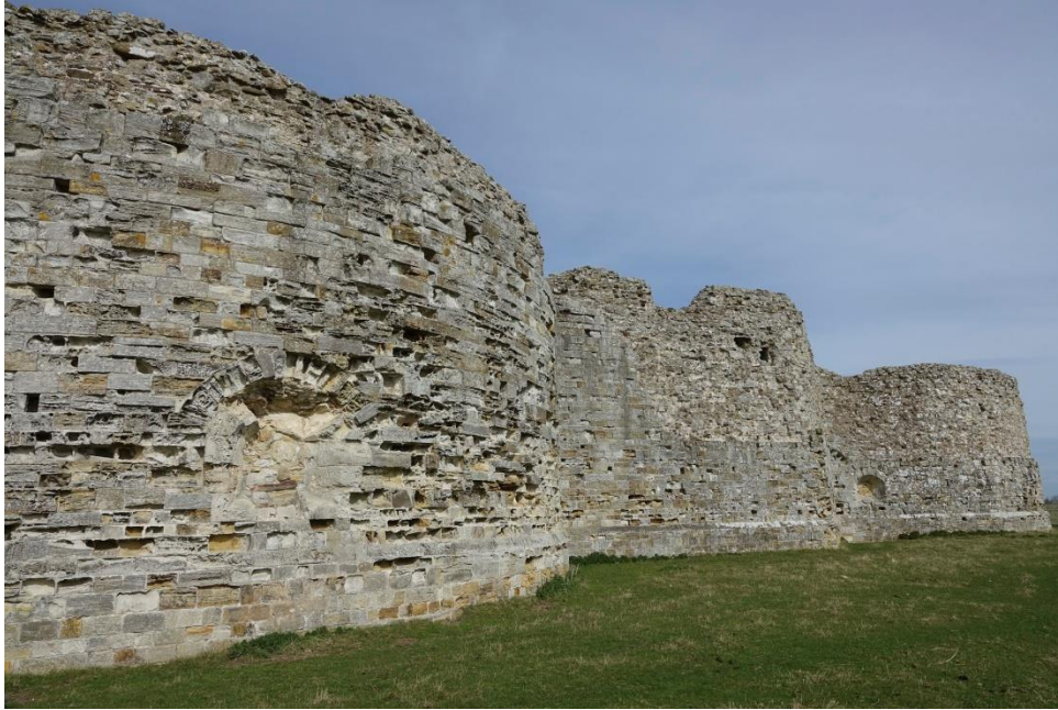
Camber Castle, Scheduled Ancient Monument – built in three phases 1512-44 on the orders of Henry VIII English Heritage site on Rye Marshes, East Sussex
