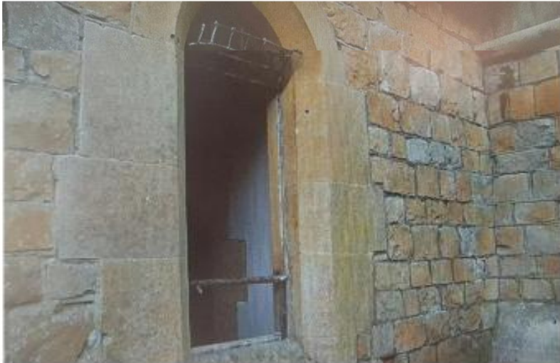
Storrington church damage. Picture: Sussex Police
