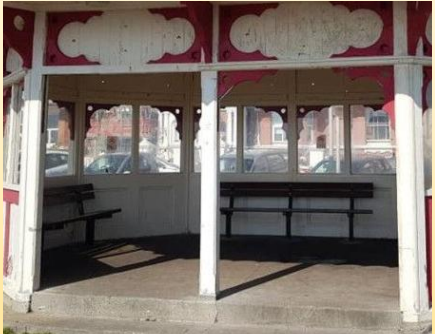
Decorative wooden panels and bench were damaged
